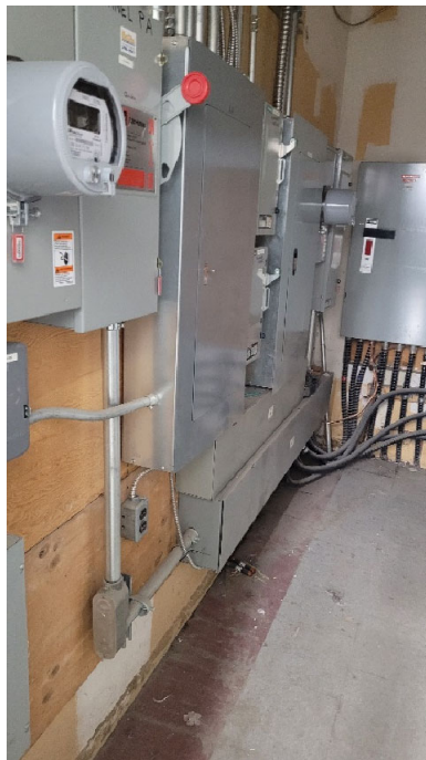
Photograph 8: View of the interior of the electrical room on the ground floor of the Site building; within Dollarama commercial unit.
