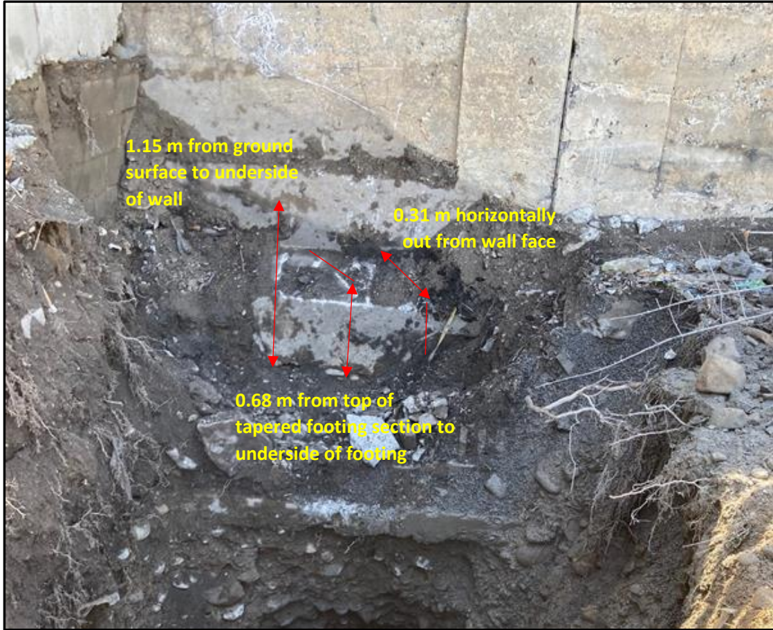
Photo 4 – Details of TP1-22, of the existing retaining wall abutment system for adjacent section of Somerset Street from field program dated April 2022. Wall abutment placed over engineered granular fill.
