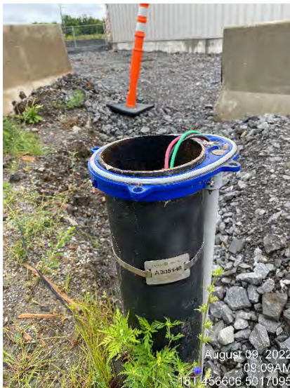
Photo 4 - Observation well (ID A305146) used during pumping test for monitoring of potential interference effects.
