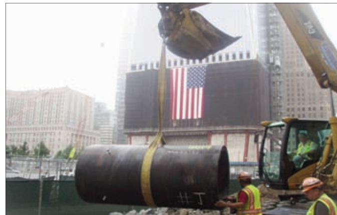
48" CheckMate® installed at the Freedom Tower for stormwater drainage.
