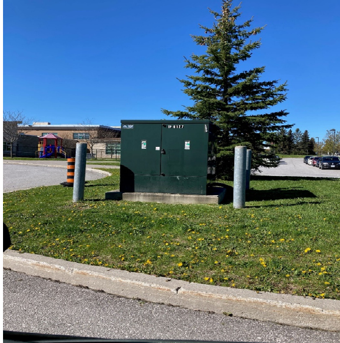
Photograph I3: Pole and pad mounted transformers identified throughout the study area.
