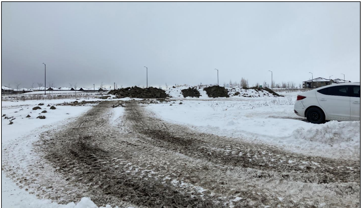
Figure 5: View of the stockpile soil on Subject Site looking southeast from Putney Crescent.
