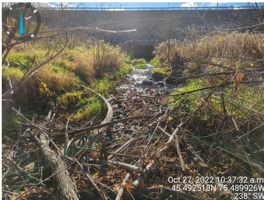
Photo 12: Taylor Creek near the upstream end, looking upstream at the culvert flowing under Highway 174 (October 27, 2022)
