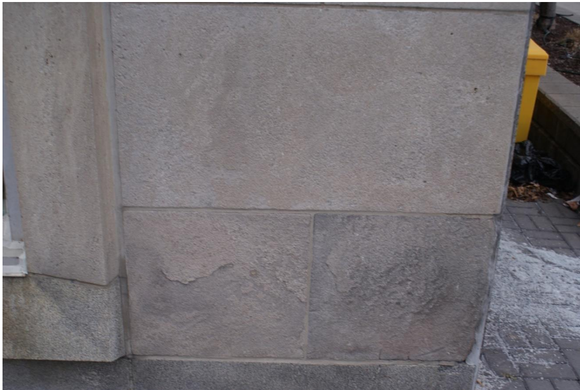
Figure 15: Detail view at the base of the wall at the south-west corner. The surface of the two Niagara limestone panels at the base of the wall are scaling due to de-icing salts. The granite plinth course is evident at the bottom of the photo. The Niagara limestone window surround is the vertical element to the left and a granite window sill/surround below. Source: Commonwealth 2022.
