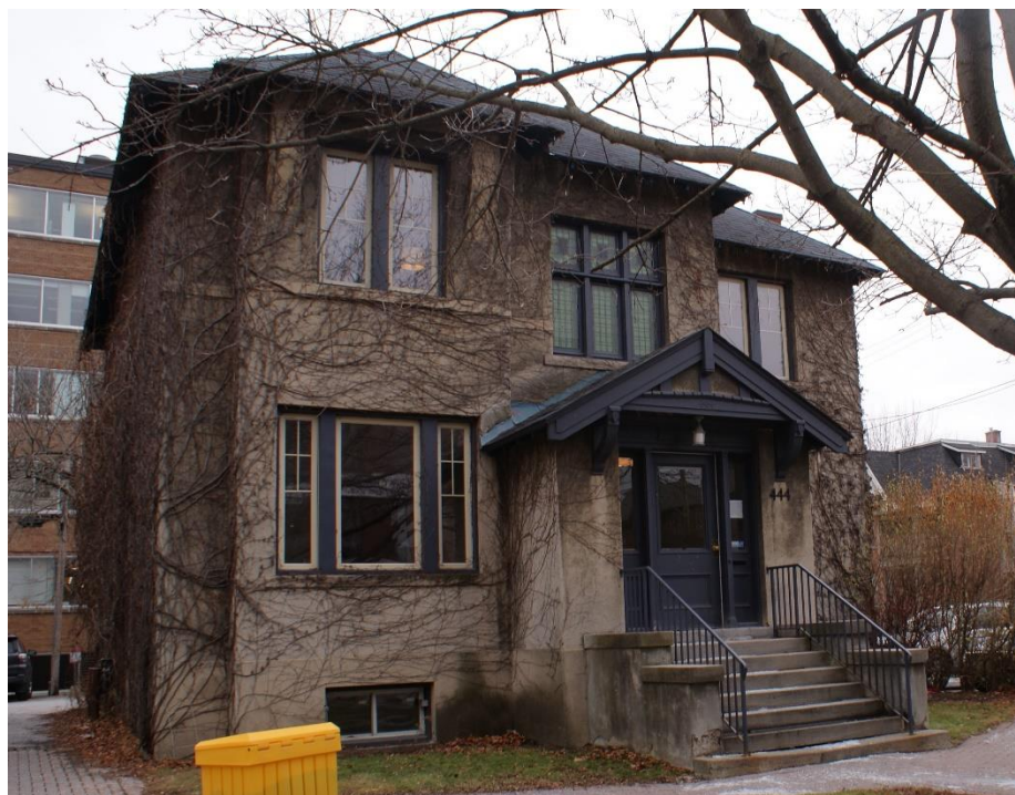
Figure 26: View of 444 MacLaren Street. The stuccoed exterior wall is covered in vines that should be removed before they have an adverse impact on the stucco finishes. Source: Commonwealth 2022
