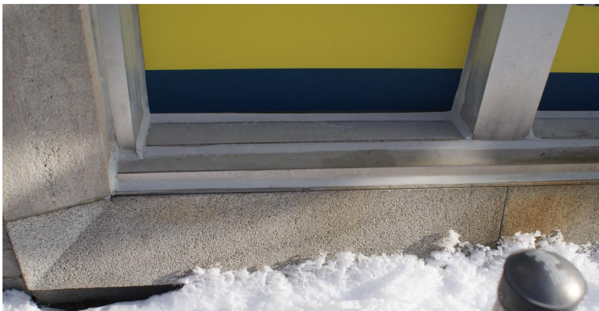
Figure 16: Detail view of the base of the Kent Street window. The horizontal units at the base of the window are formed of the same material as the granite plinth course. The vertical stone to the left is a limestone unit. Note the close match in colour and surface texture. Source: Commonwealth 2023
