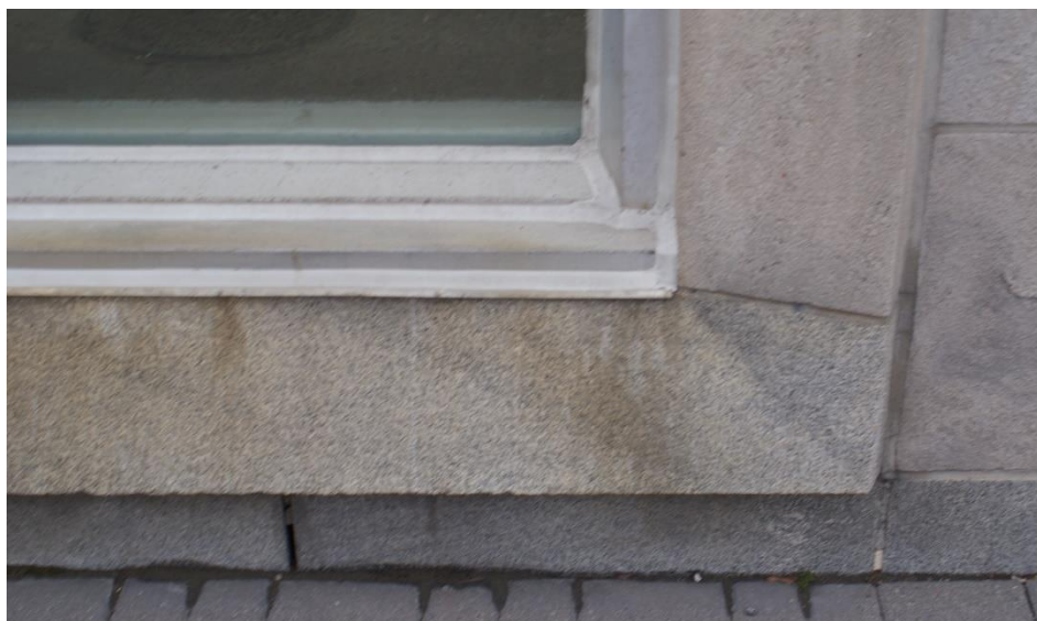
Figure 18: Detail of the granite plinth course and granite windowsill surround at the base of the three-storey Kent Street window. The colour of the granite sill is very close to the limestone cladding and window surrounds. Source: Commonwealth 2022.
