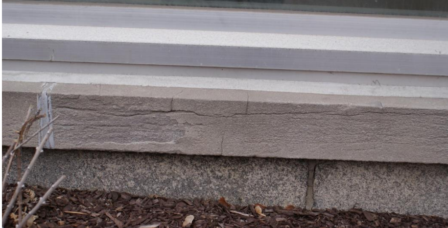
Figure 13: View of a deteriorated limestone windowsill and the granite plinth course below. The cleavage planes within the limestone sills are evident where the sawn surface has weathered. The cleavages planes follow the layers of deposition of the sedimentary rock. Source: Commonwealth 2022.
