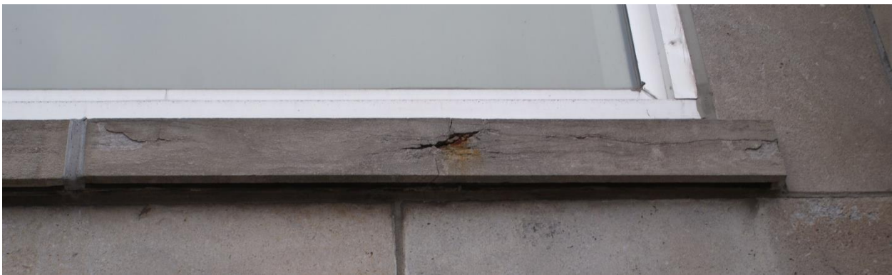
Figure 14: View of a deteriorated limestone windowsill. The cleavage planes within the limestone sills are evident where the sawn surface. The cleavages planes follow the layers of deposition of the sedimentary rock. Source: Commonwealth 2022.
