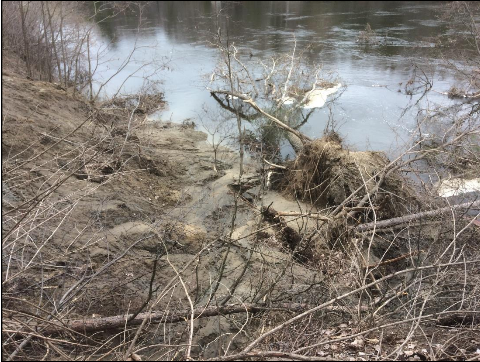
Photo 3: Slope toe in failure area along Rideau River at same location as noted in Photo 2.
