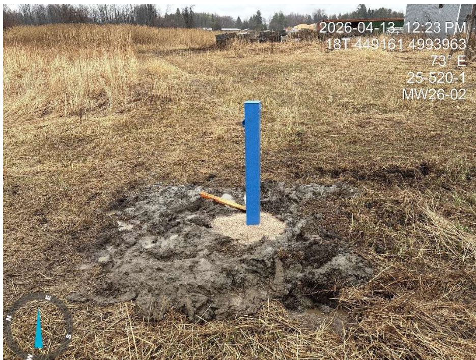
Photograph 2: Photograph of installed MW26-02.
