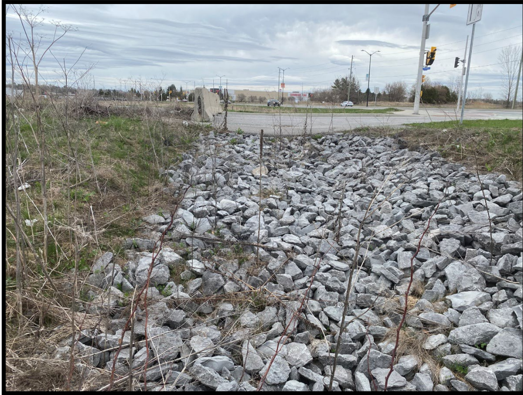
Figure 11: Example of disturbed conditions (MH1446-D035).
