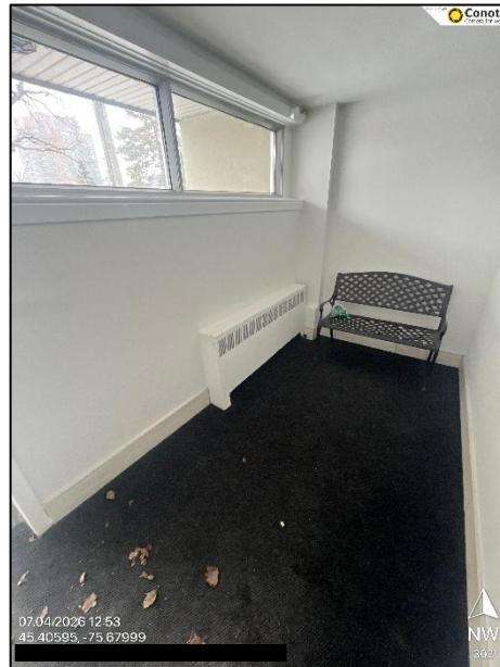
Example of the heating units observed throughout the on-site residential building
