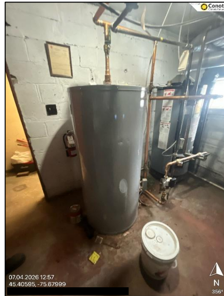
Water heater observed in the mechanical room in the western portion of the on-site residential building
