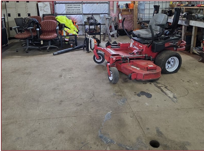
Photograph K9 – Looking south inside shop. Use for storage of equipment and small quantities of oil. Minor staining on the concrete flooring along with a drain.
