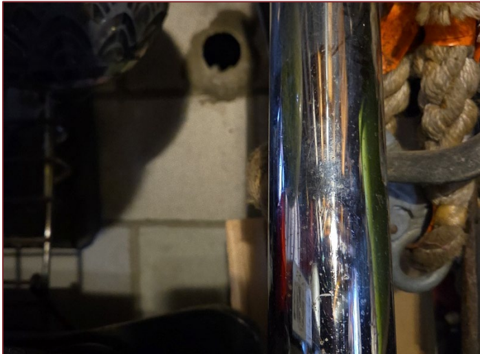
Photograph K15 – Looking west inside the residential building basement. Hole in the wall likely for the piping for the historic UST.
