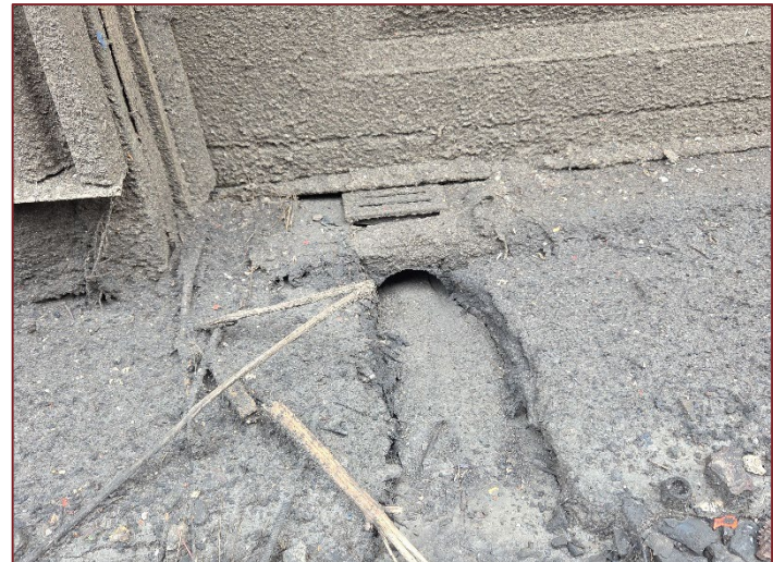
Photograph K4 – Looking north, outside of the southern side of the small shop at the exit of the interior drain.
