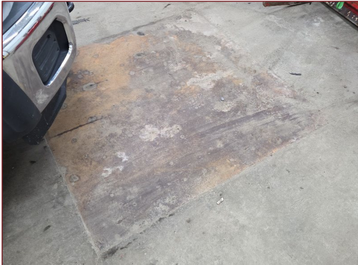
Photograph K3 – Looking south inside the small shop. A cut area of the concrete floor where the water well is expected to be located.
