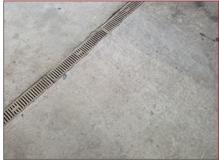
Photograph K2 – Look east inside the small shop. A drain on the concrete floor is seen.
