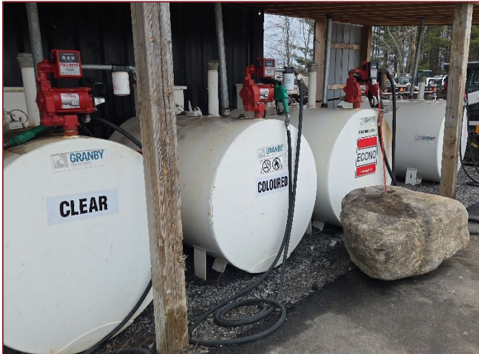
Photograph K11 – Looking east at multiple ASTs under a roofed structure. ASTs are located directly on the gravel flooring. No staining was observed.
