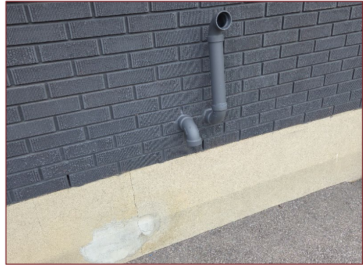
Photograph K14 – Looking east at the side of the residential building with a historic fill and vent pipe for the historic UST.
