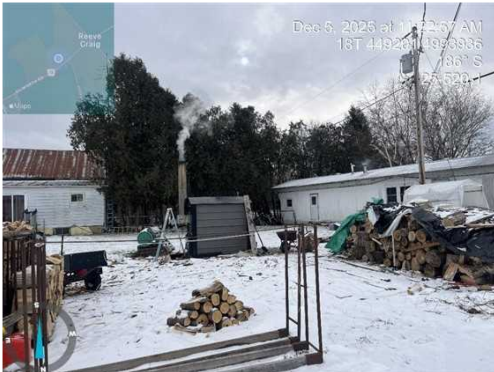
Photograph 17 – Exterior wood burning stove.
