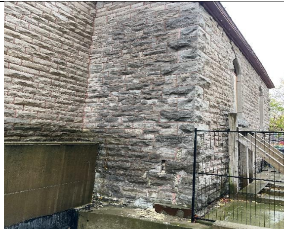
Photo 9: Bulge on north wall of Annex. Wall is braced. Little evidence of movement in past two years.
