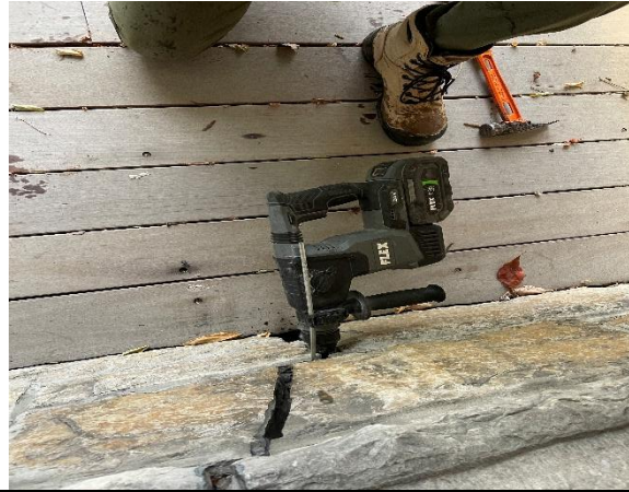
Photo 4: East wall of House. Fracture at window. Hard grey Portland pointing mortar. Sand and voids in fracture.
