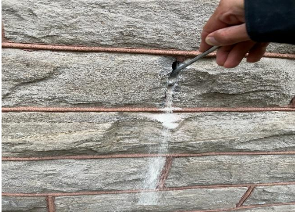
Photo 3: West wall of Convent. Hard pink Portland pointing mortar still bonded to stone. Back up mortar is reduced to sand.
