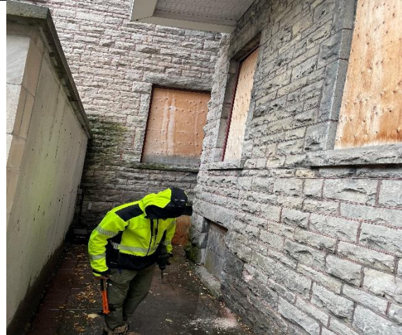
Photo 6: East chapel wall. Condition as Photo 4. Sand in joints up to 250mm deep.
