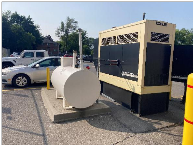
Photo 8 – Photo of generator and associated diesel AST located on the north east portion of the Phase One Property, looking south.
