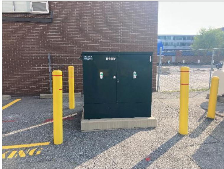
Photo 7 –Photo of transformer located on the northeast portion of the Phase One Property, looking east.
