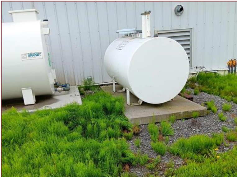
Photograph L11 – Looking south towards the diesel storage tank on concrete slab.
