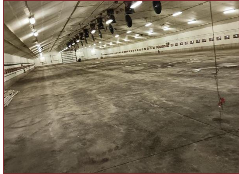
Photograph L6– Looking west inside the barn. Slab floor on grade. Venting overhead and vent windows along wall. Some staining from agricultural practices.
