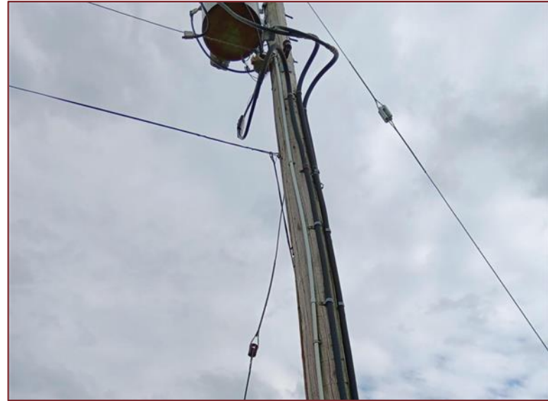
Photograph L14 – Looking north, up the pole. An electrical transformer on the pole with no staining seen on the wood below it..
