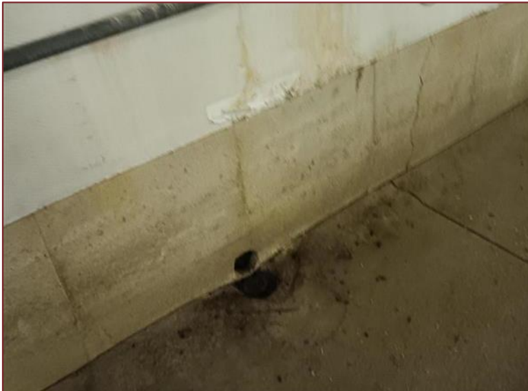
Photograph L7 – Looking north inside the bar. A drain located at the intersection of wall and floor. Multiple drains are within the barn. Piping for water above drain and below venting window.
