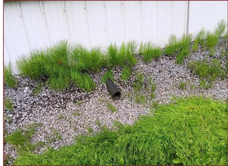
Photograph L10 – Looking south at the barn. Drain exit from the inside of the barn
