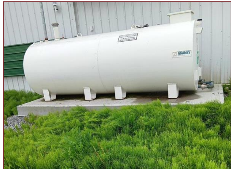
Photograph L12 – Looking south towards the furnace oil storage tank on concrete slab.
