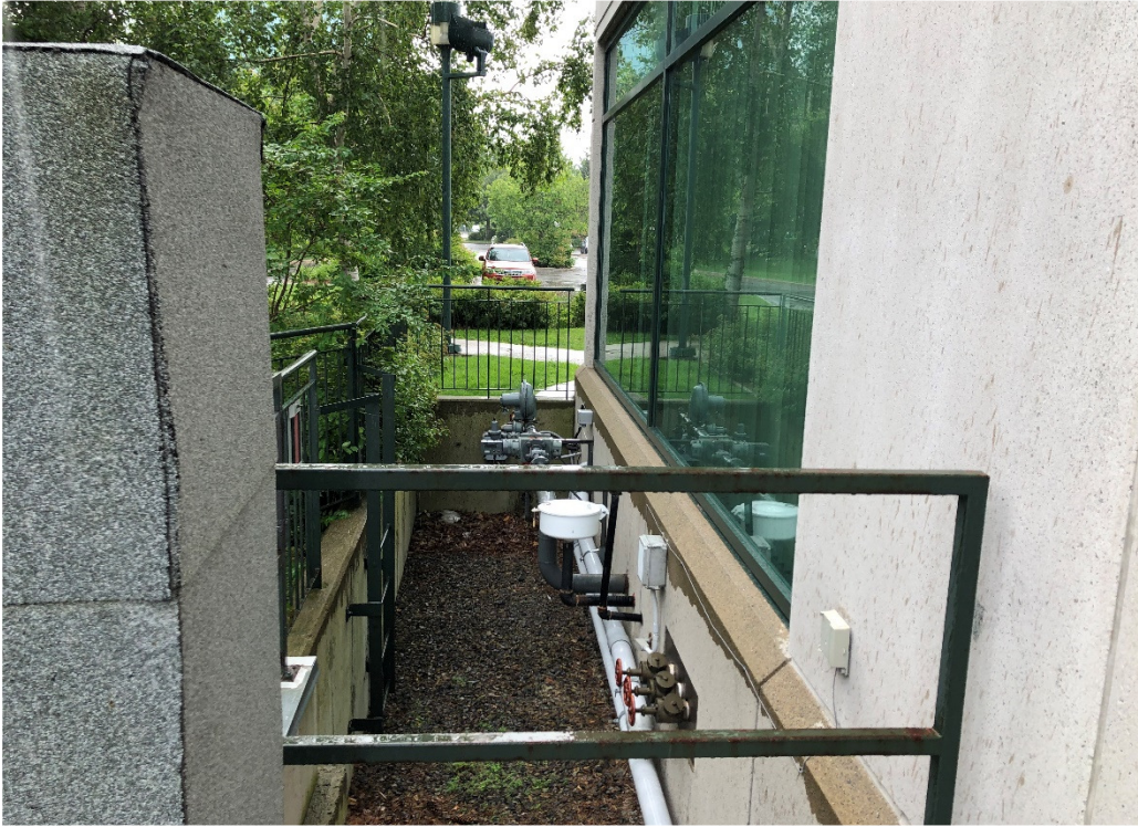
Photograph 3: Location of vent and fill pipes for associated AST, on eastern side building.
