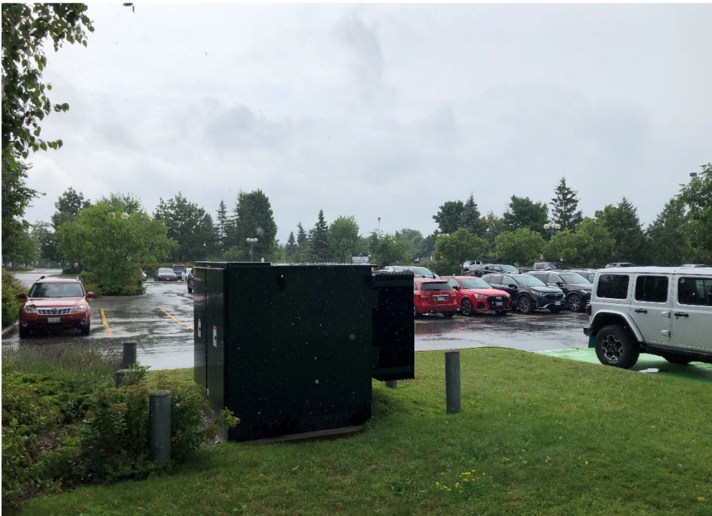
Photograph 4: Pad mounted transformer located at the southern side of 535 Legget Drive.
