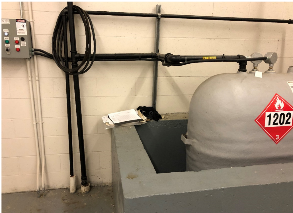
Photograph 2: AST located in the mechanical penthouse of 535 Legget Drive.
