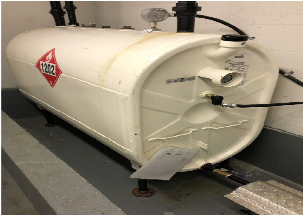
Photograph 1: AST located in the basement of the 535 Legget Drive, in the southeastern corner of the building.
