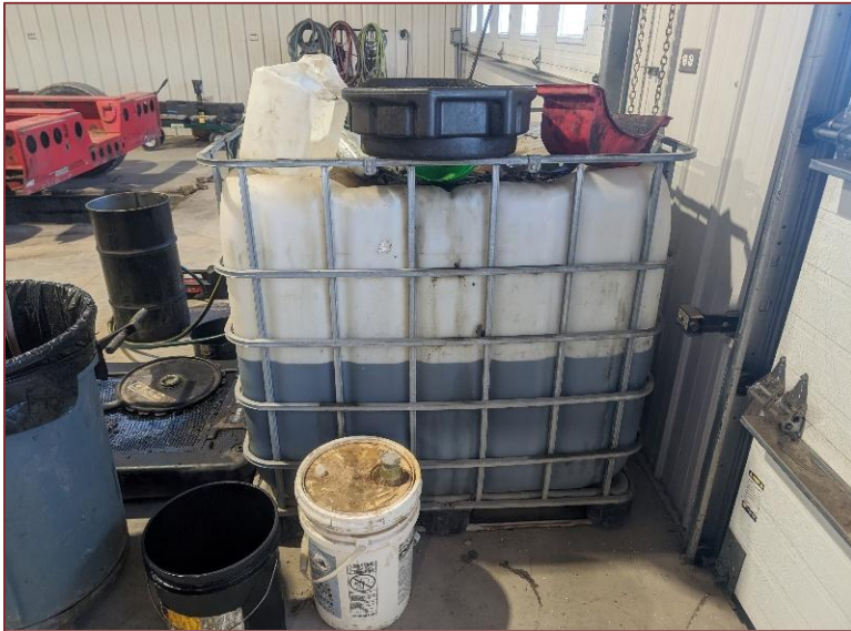
Photograph L11 – Looking east inside the Structure 7 (Building Workshop). An oil tote was present inside the Structure 7. No signs of spills, staining or odors were noted at this location.
