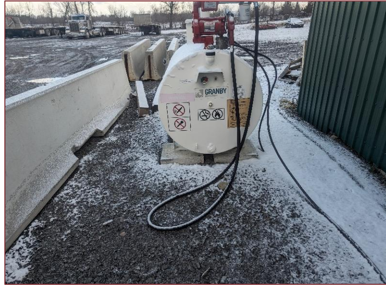
Photograph L18 – Looking north at one of the ASTs along the west building line of Structure 3 (Material Storage). The ASTs were in good working condition and there were no signs of spills, staining or odors were noted at this location.
