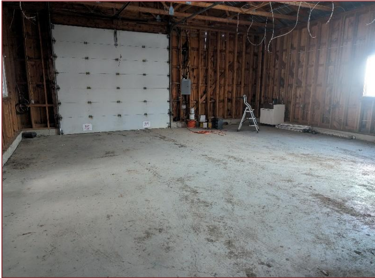
Photograph L21 – Looking north inside Structure 6 (Sales Shop). Concrete flooring was in a good shape with minimal cracking.
