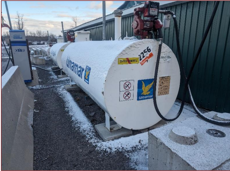
Photograph L17 – Looking north at the ASTs along the west building line of Structure 3 (Material Storage). The ASTs were in good working condition and there were no signs of spills, staining or odors were noted at this location.
