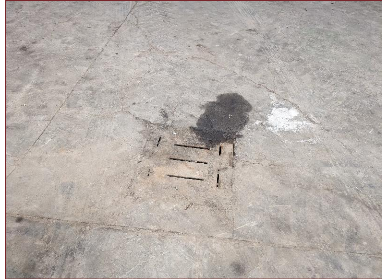
Photograph L14 – Looking west inside the Structure 7 (Building Workshop). A photo of the drain.
