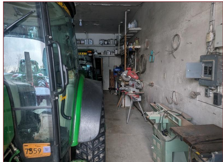
Photograph L16 – Looking north inside the Structure 3 (Material Storage). Concrete flooring was in a good shape with minimal cracking. No signs of spills, staining or odors were noted at this location.
