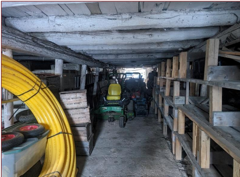
Photograph L15 – Looking north inside the Structure 3 (Material Storage). Concrete flooring was in a good shape with minimal cracking. No signs of spills, staining or odors were noted at this location.
