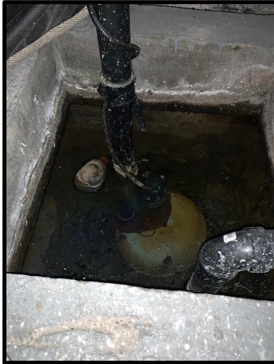
Photograph 5: View of the sump pit with sheen located in the basement of the 1137 Ogilvie Road.
