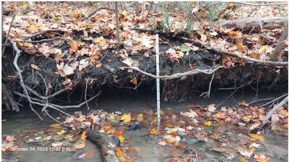
Photograph taken facing the right bank at the downstream extent of the reach. Undercutting was not commonly observed with exception to the outside bend along the downstream extent of the reach where undercutting was measured up to 1.05 m.
