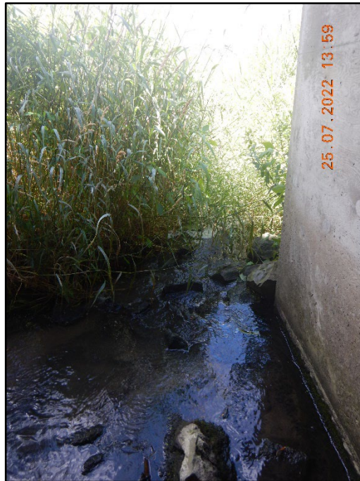
3. Wilson Cowan Drain - Facing downstream from inside culvert, the flow path is to the right side of the culvert flowing into a defined channel
