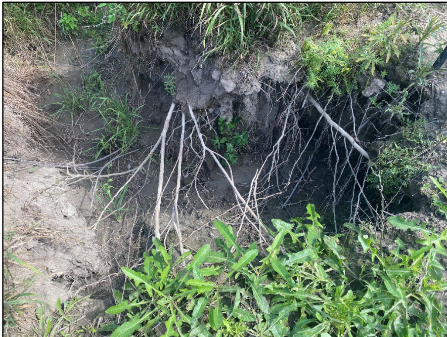
16. Mud Creek– Drainage from the adjacent field has resulted in a significant washout along the southern bank of Mud Creek
