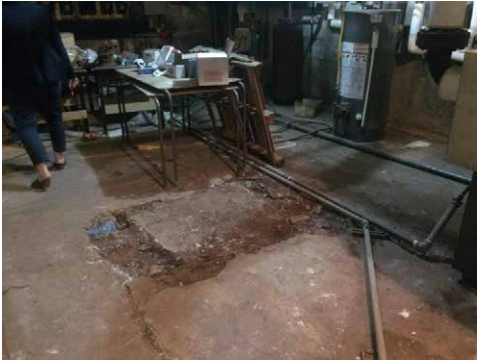
Photograph 13. View of the mechanical room, located in the basement of the church
