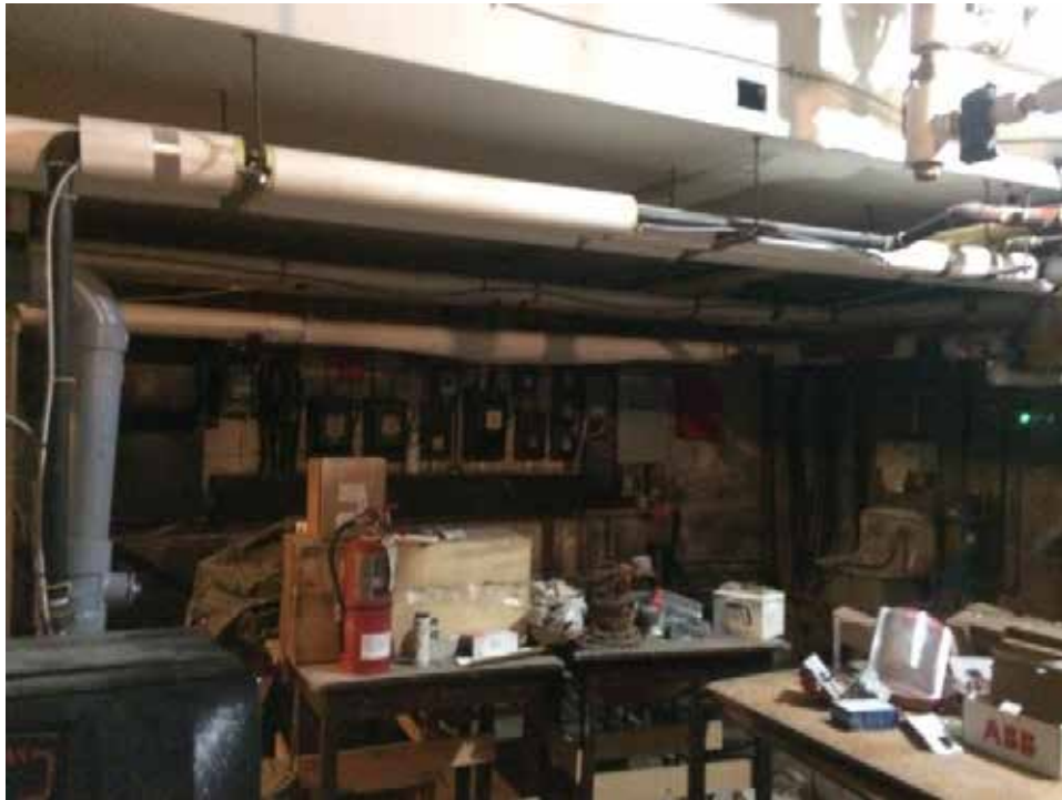
Photograph 11. View of the mechanical room, located in the basement of the church
