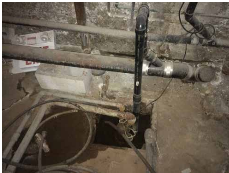
Photograph 15. View of a sump pit, located in the mechanical room of the church
