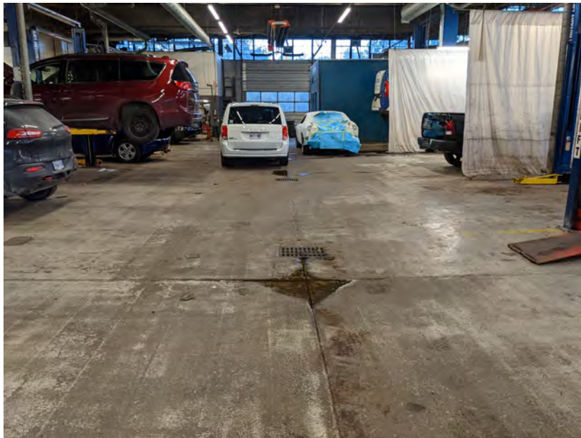
Photo 14 – Garage driveway, drains located in the center of the garage along the length of the floor. Looking north
