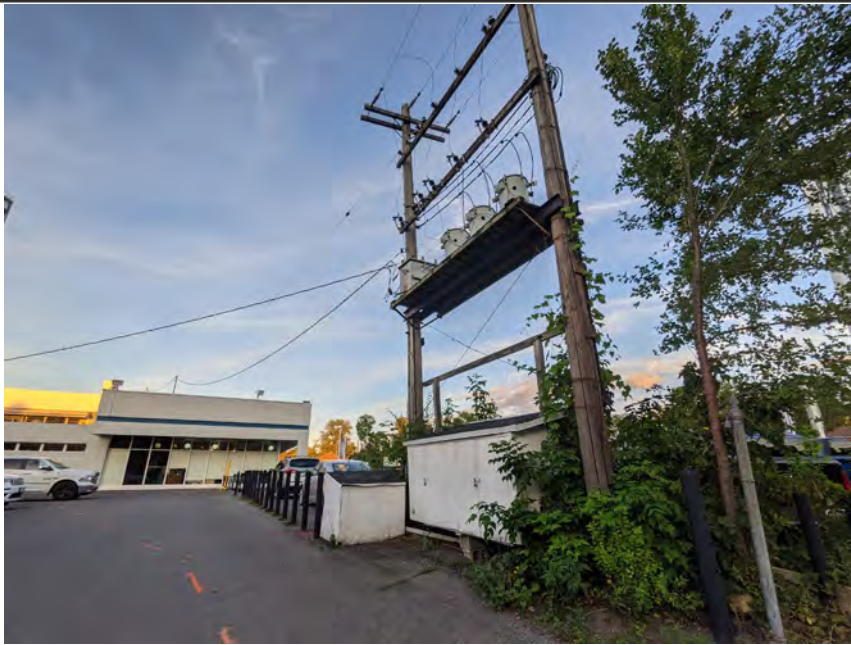
Photo 11 - Suspended transformers, westside parking lot entrance, adjacent to New Orchard Ave, facing northeast
