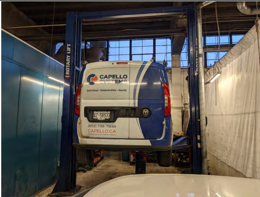
Photo 21 - Hoists in the garage, along the eastside
