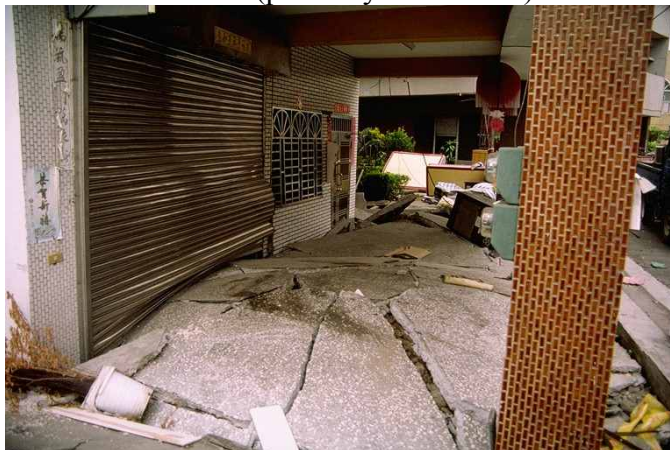
(c) Close-up view of foundation failures beneath a building [seen on left side of photo (a)] near the locations of borings WAS-3 and WAS-4 (photo by R. B. Seed)
