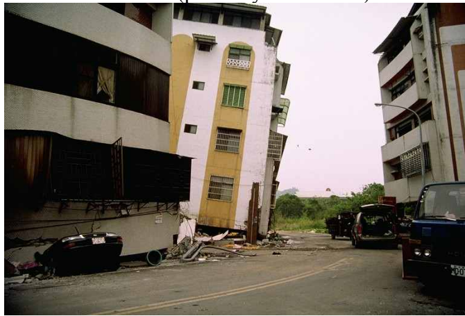
(b) 5- and 6-story buildings with foundation failures near the locations of borings WAS-3 and WAS-4 (photo by R. B. Seed)
