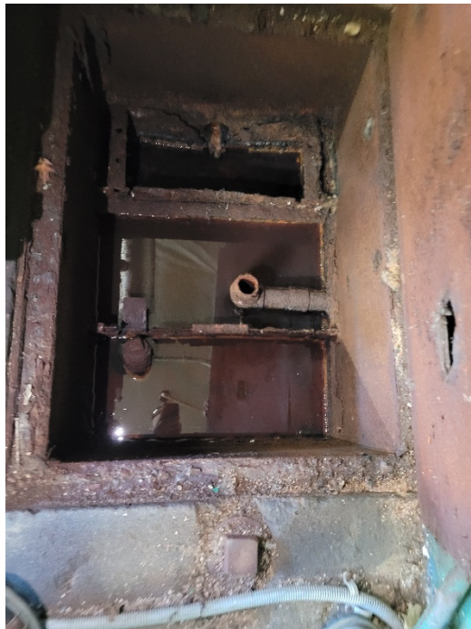
Photograph 6: View of the interior of the oil/water separator in the service bay of the building at the Property. An oily water mixture is evident within the separator.
