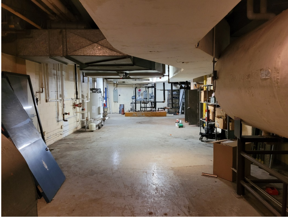
Photograph 7: View of the basement level mechanical room in the east portion of the building. The sump is visible at the rear wall in this photograph.
