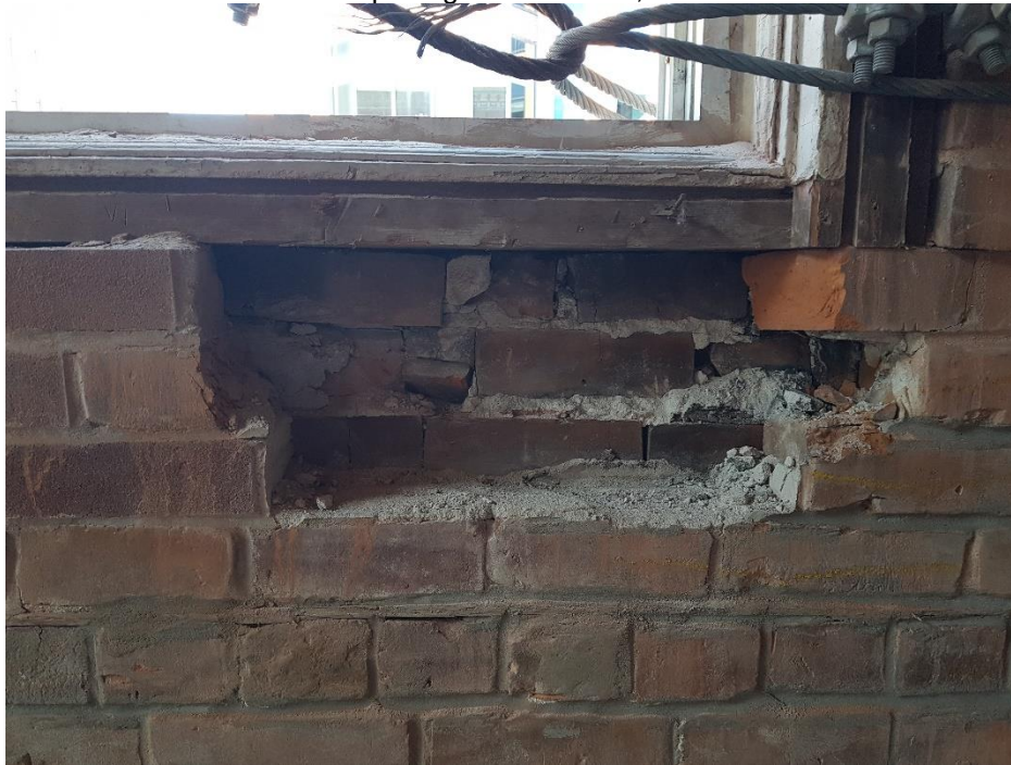
Photograph 12: View of the middle wythe condition. Mortar in poor condition and some cracked bricks. Opening on north wall, second floor (below window to extract middle wythe).
