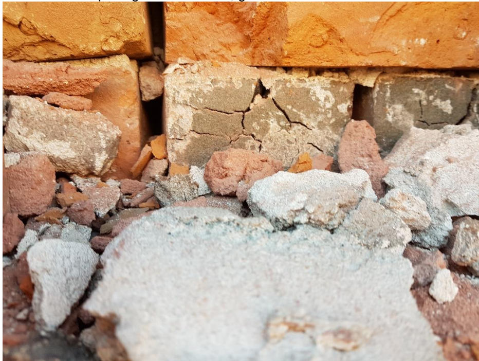
Photograph 14: Close-up view of the middle wythe condition. Mortar deteriorated, crack and crushed bricks. Opening on the exterior, ground floor of the north elevation.
