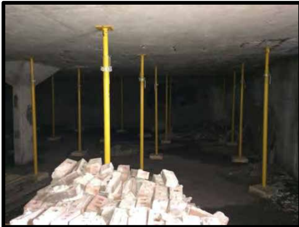
Photograph 2: View of interior of lower portion of the parking structure, facing east from the western portion of the structure. Some debris and bricks are present in the foreground.
