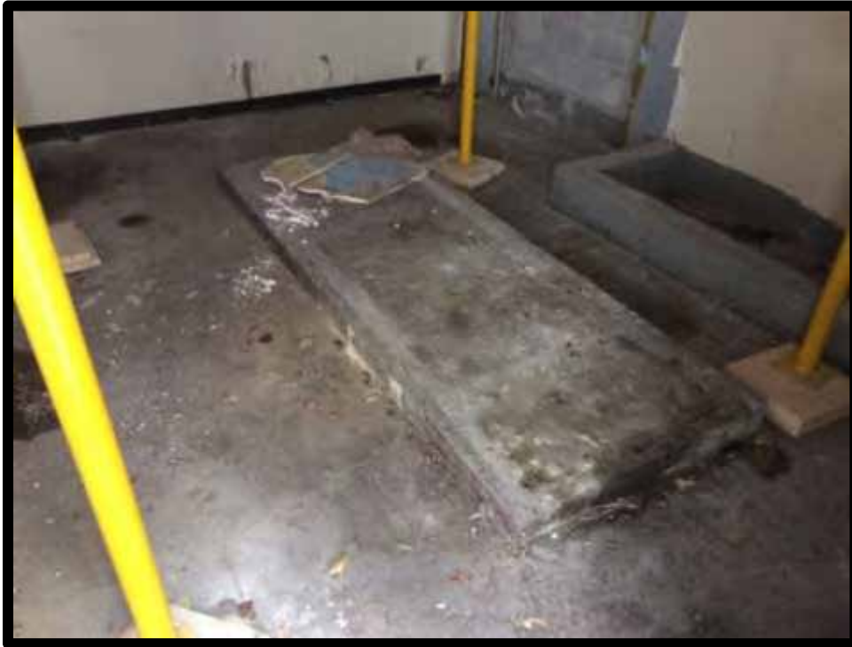
Photograph 1: View of former generator room. The concrete slab and berm are evidence of the former generator and tank locations. Concrete was observed to be in good condition with minimal staining.
