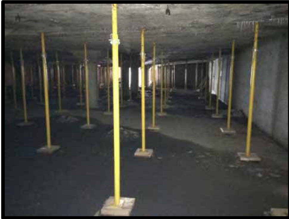
Photograph 3: View of the interior of the lower level of the parking structure. Facing west from the eastern end of the structure.
