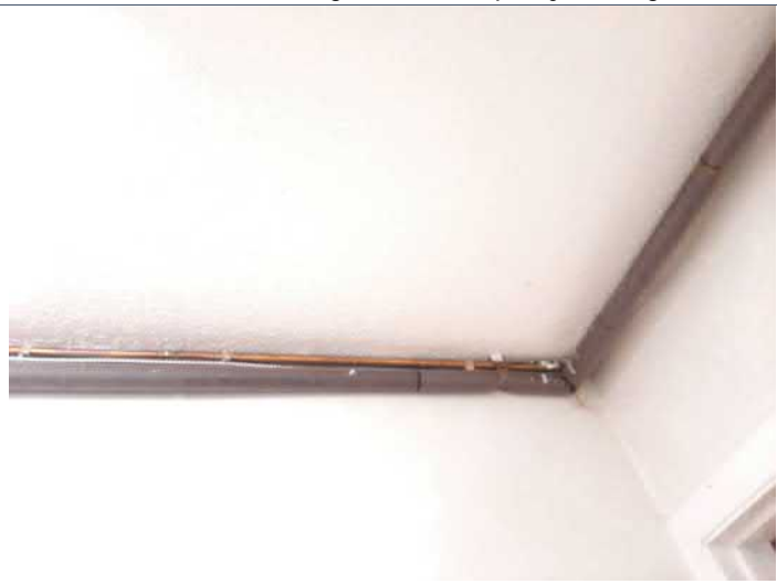
Picture 3 – Piping inside site building
