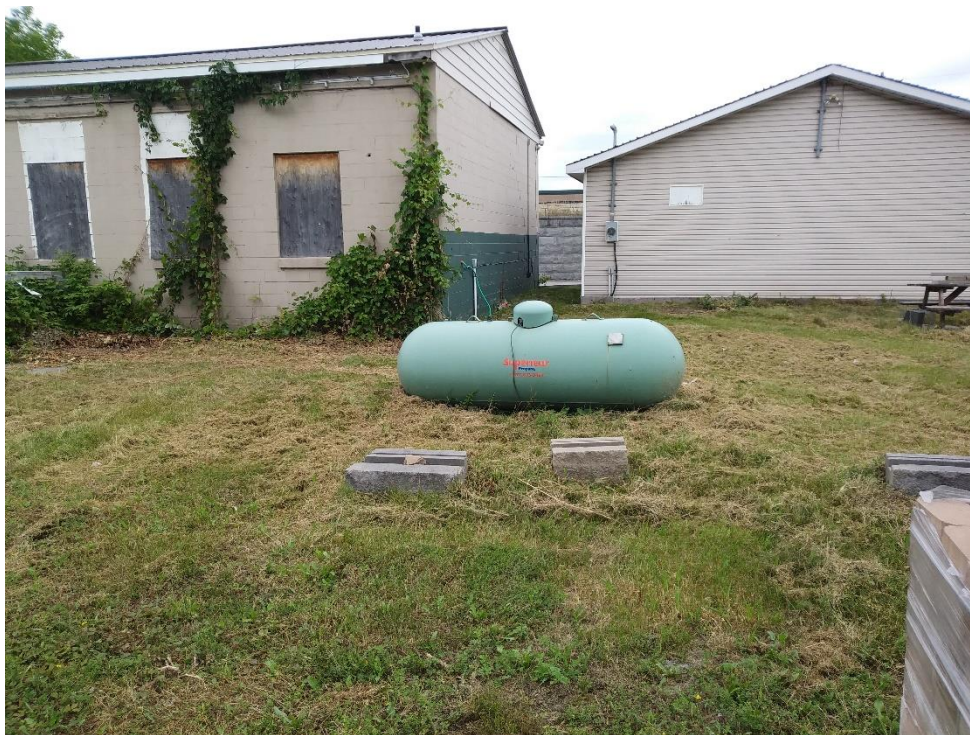
Photo 10: Propane above ground storage tank, behind office building
