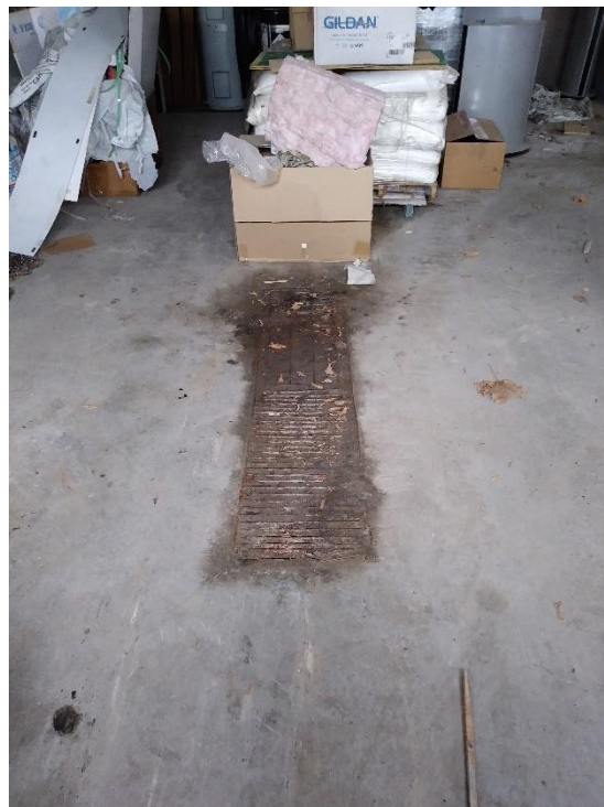
Photo 4: Pit in garage, filled in with gravel.
