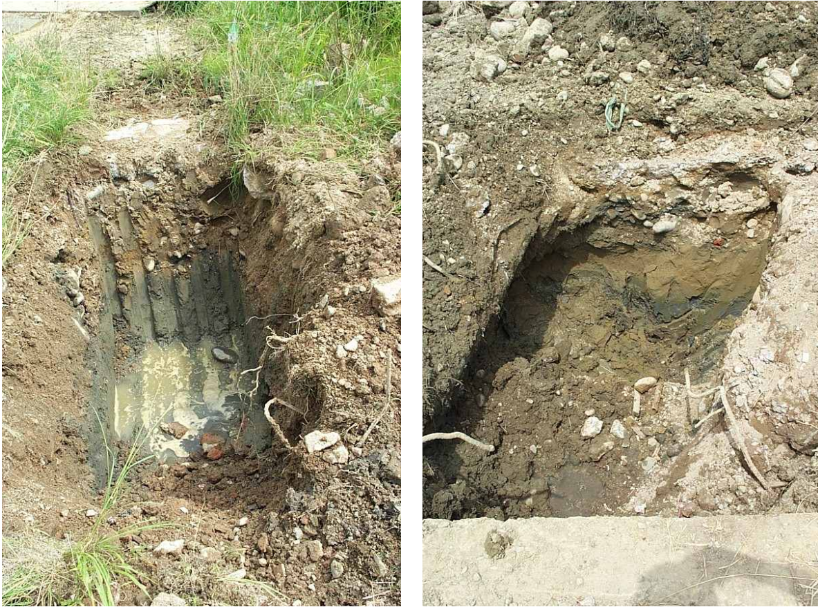
FIG. 4-27: Photographs of test pits for vane shear tests VST-3 and 4 that show the characteristics of the surface fill and underlying fine-grained soils. (source: http://peer.berkeley.edu/lifelines/research_projects/3A02/ )
