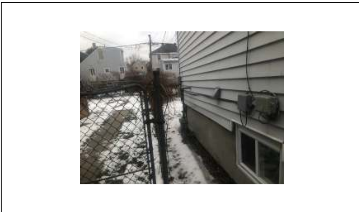
Photograph 4: Gas meter located at the north-west corner of 79 Ste-Cecile.
