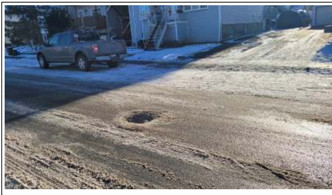
Photograph 14: View south-east of sanitary manhole in center of Ste-Cecile located in front of 73 Ste-Cecile.
