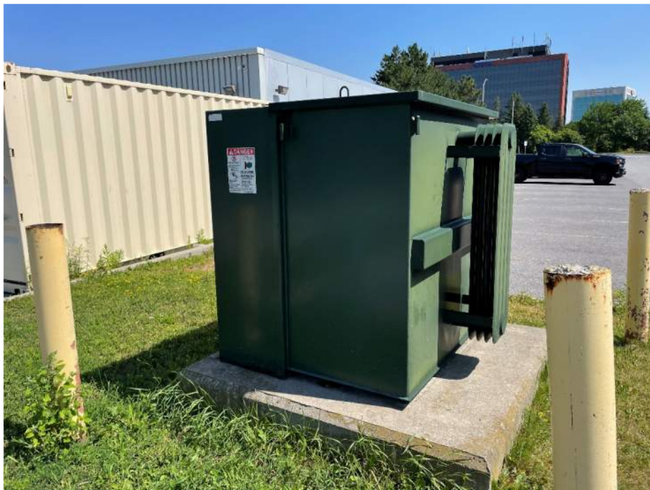
Photo 16: Transformer supplying power to the 555 March Road building. Unknown filling.
