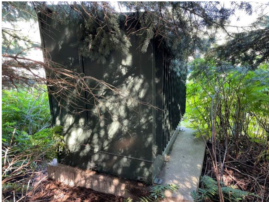
Photo 14: 2001 manufactured pad mounted, oil filled transformer along northern property boundary.
