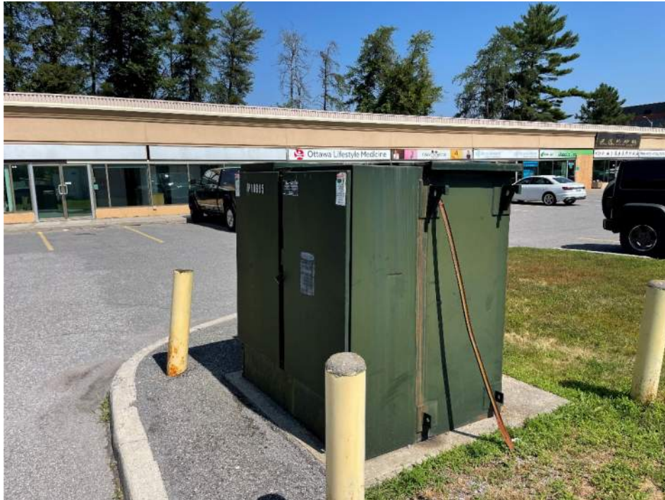
Photo 15: Transformer supplying power to the 591 March Road commercial plaza. Unknown filling
