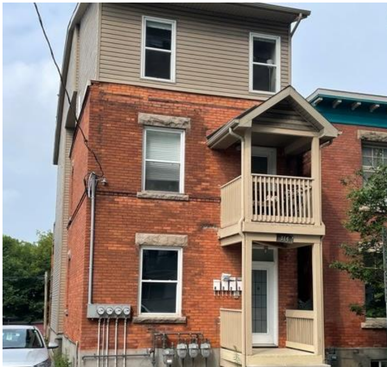
Photograph 1: View of the east side of the subject building, taken from Bell Street South.
