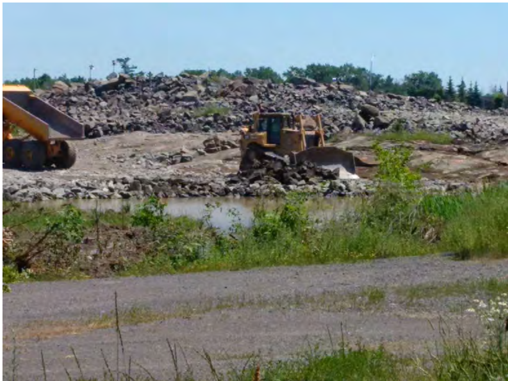
Photo 2 : Filling in a depression on west side of site with ripped bedrock.
