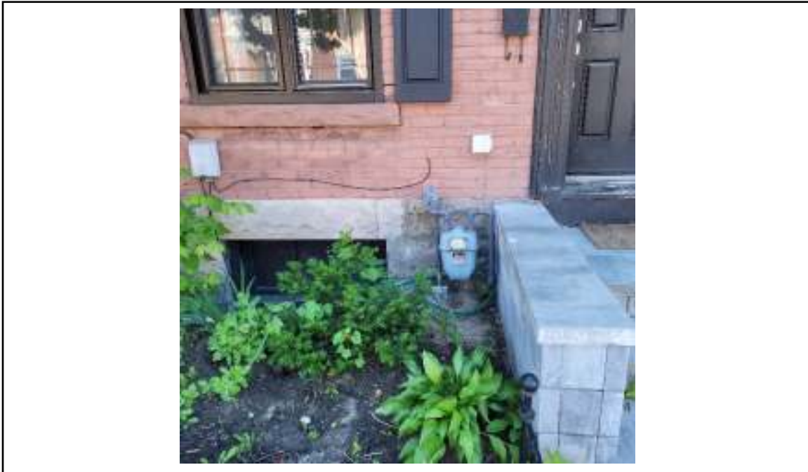
Photograph 29: Looking south at natural gas service for 16 Hawthorne.
