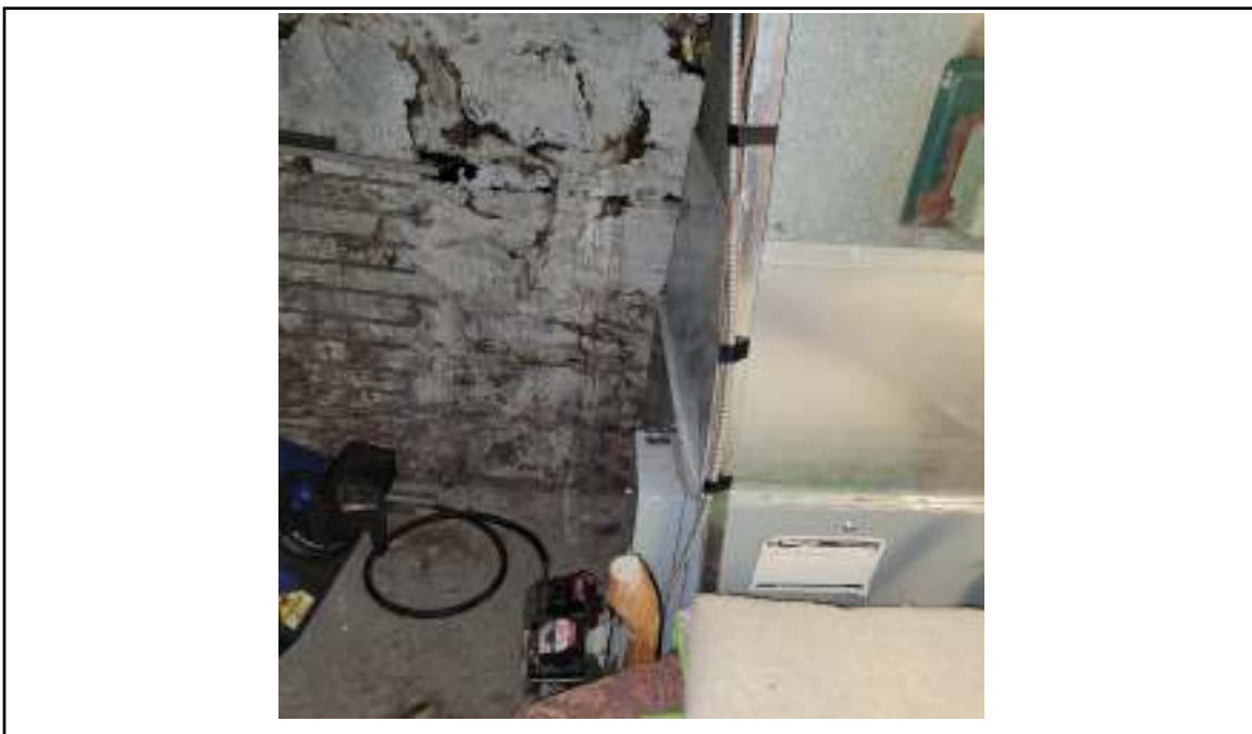
Photograph 22: Oil fired furnace in south end of basement of 18 Hawthorne.
