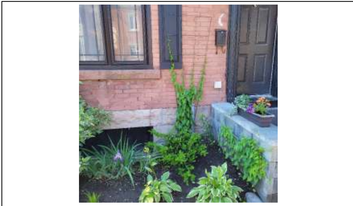
Photograph 5: Looking south at north front wall of 18 Hawthorne, note fill and vent pipes for AST in basement of unit.
