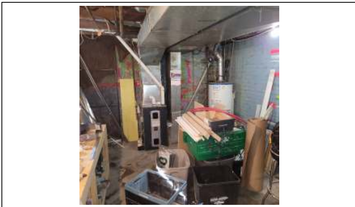
Photograph 6: Natural gas furnace and hot water tank in basement of 14 Hawthorne.
