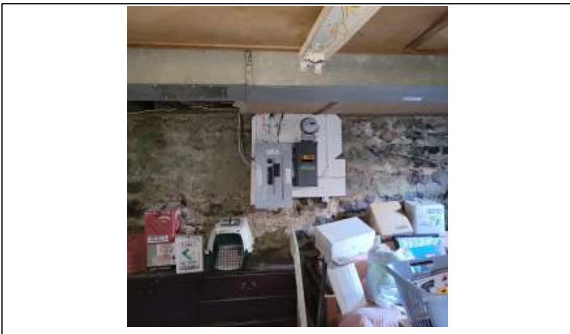
Photograph 10: Main electrical panel in basement of 12 Hawthorne.
