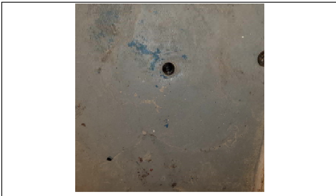
Photograph 16: Floor drain in floor of basement of 16 Hawthorne.
