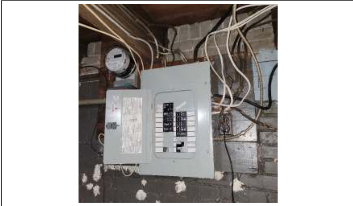
Photograph 7: Main electrical panel in basement of 14 Hawthorne.
