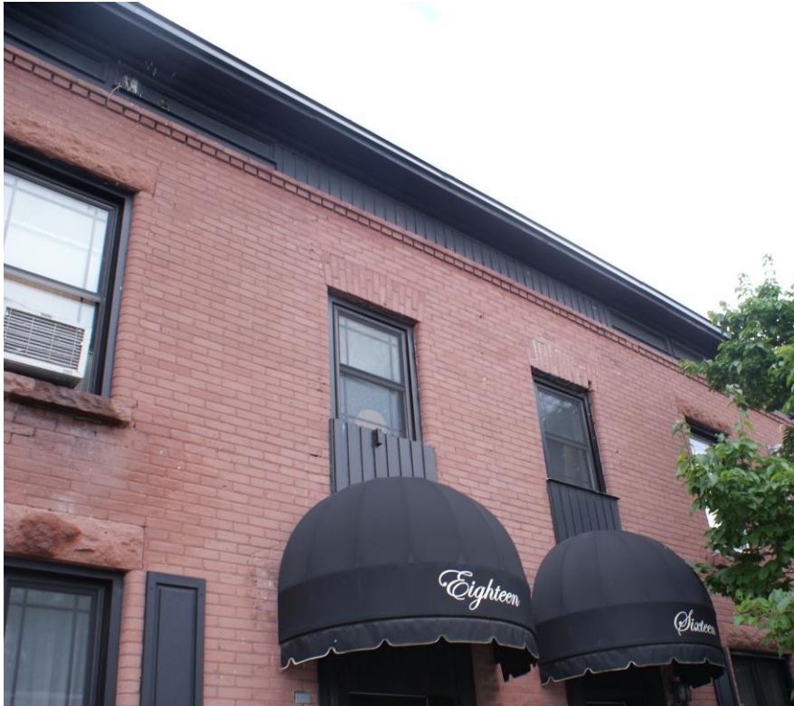
Figure 12: View of the altered second floor doors, stringcourse detailing and alterations to the cornice band. Source: Commonwealth
