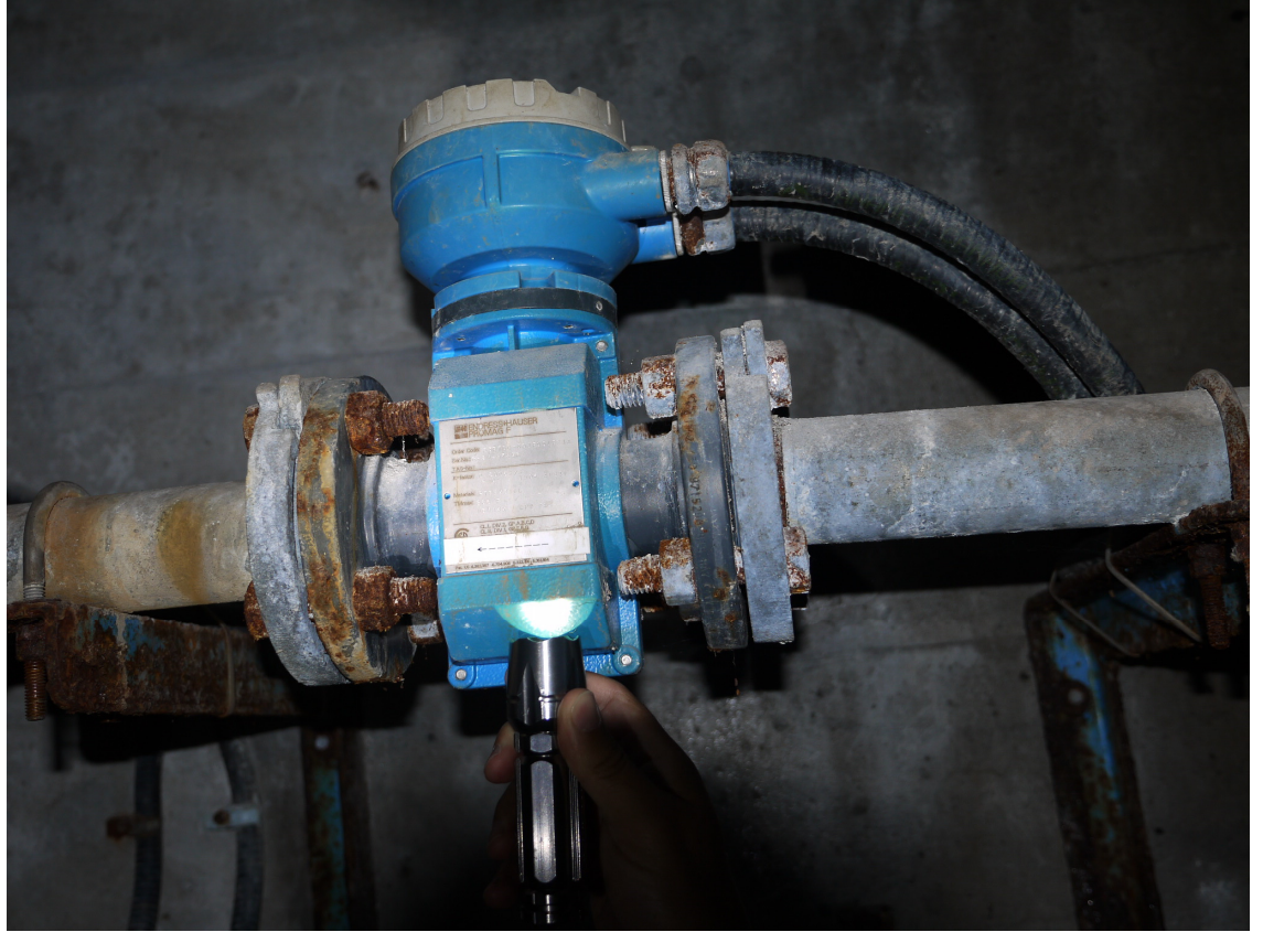
Photo 1: Flow meter: Endress + Hauser ProMag F
