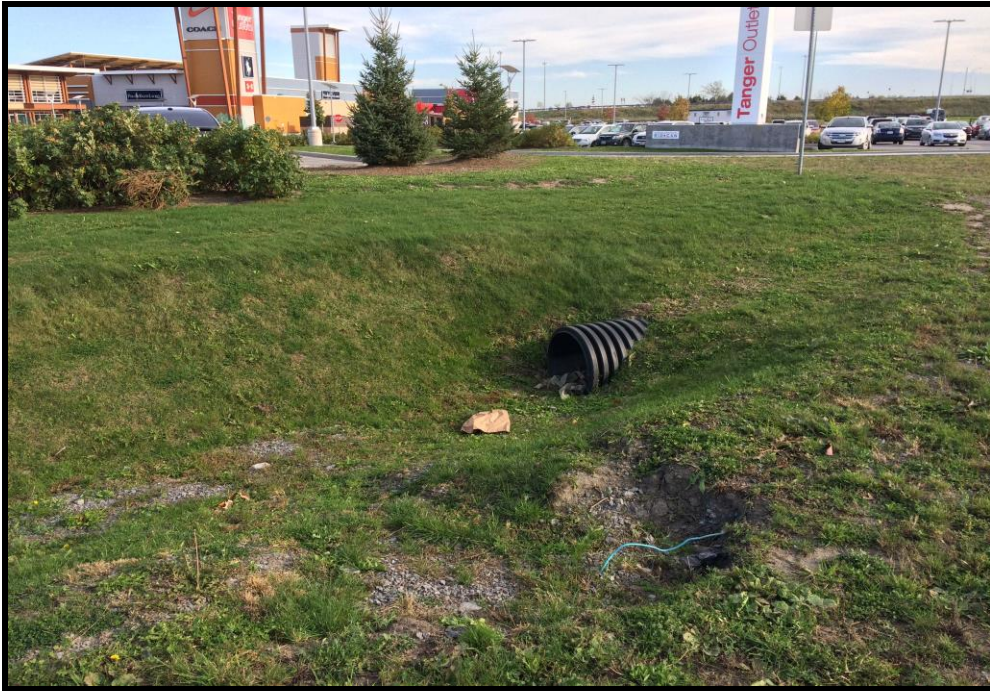
Photograph 5: View of a drainage culvert located in the eastern portion of the property, facing southeast.
