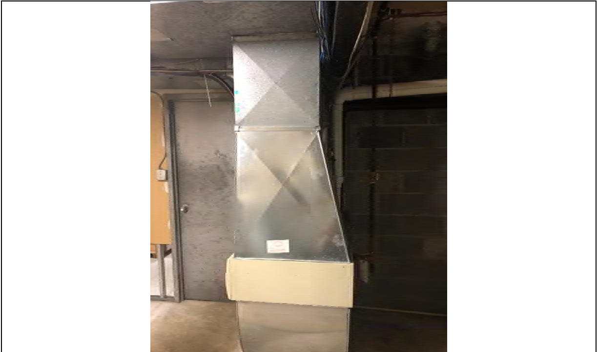
Photo 003 View of HVAC system in the basement of the building on the Site (facing north).
