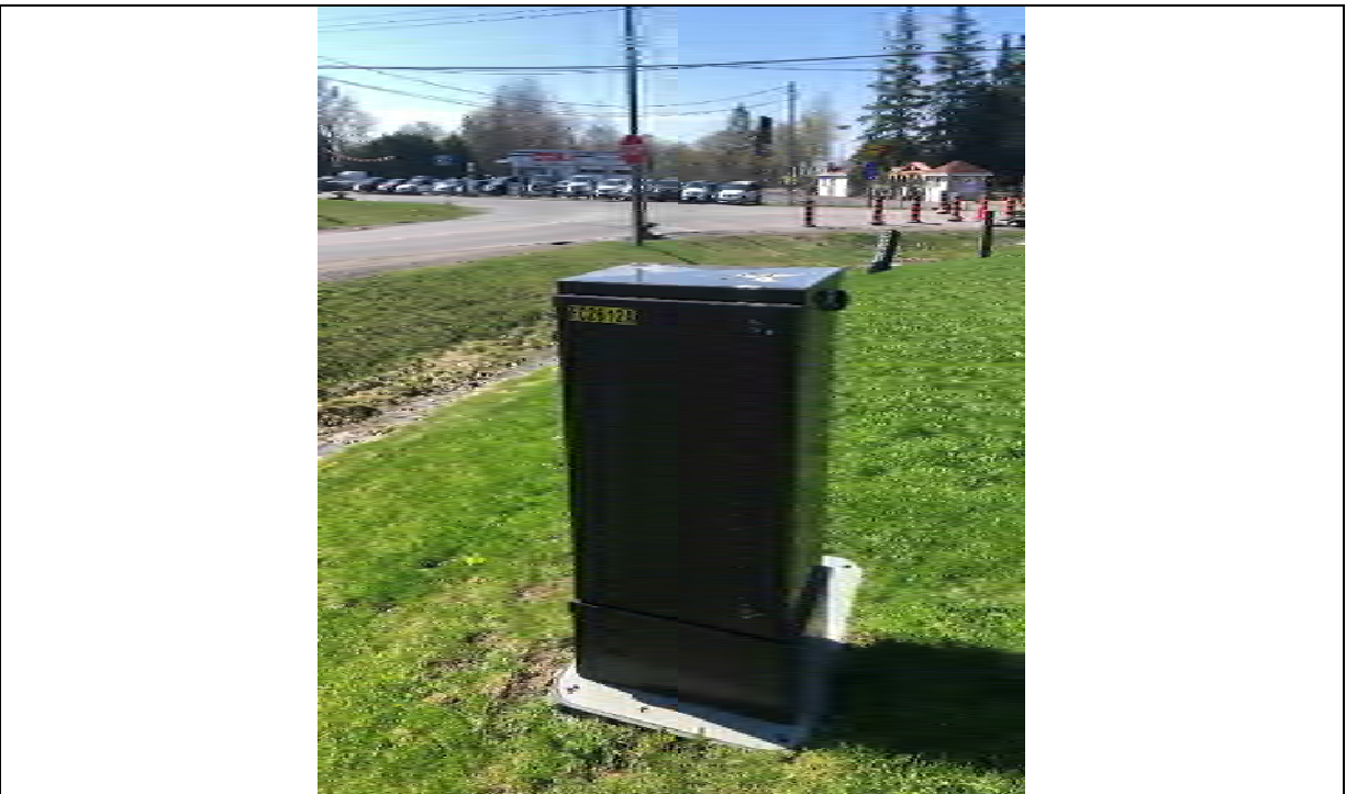
Photo 008 View of a transformer on the Site, with the intersection of Navan Road and Mer Bleue Road in the background (facing southeast).
