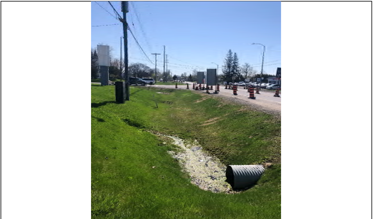
Photo 010 View of ditch along the southern Site boundary including a culvert under Navan Road (facing east).
