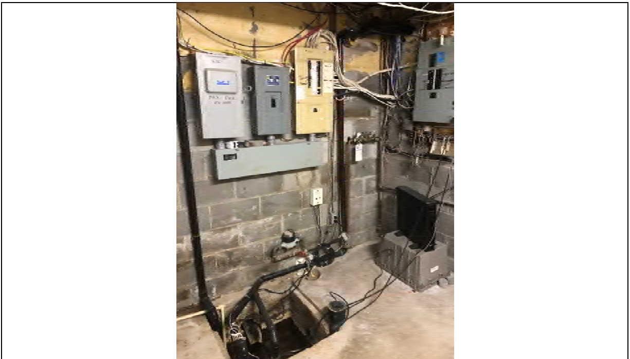
Photo 004 View of sump in the basement of the building on the Site (facing southwest).
