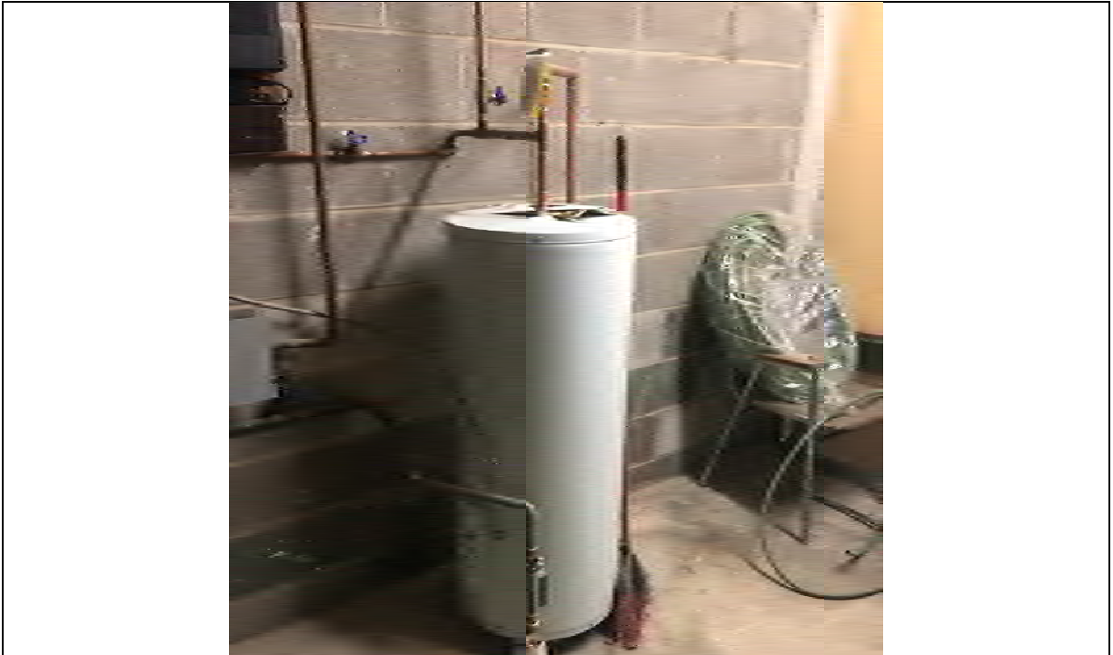
Photo 005 View of hot water tank in the basement of the building on the Site (facing southeast).
