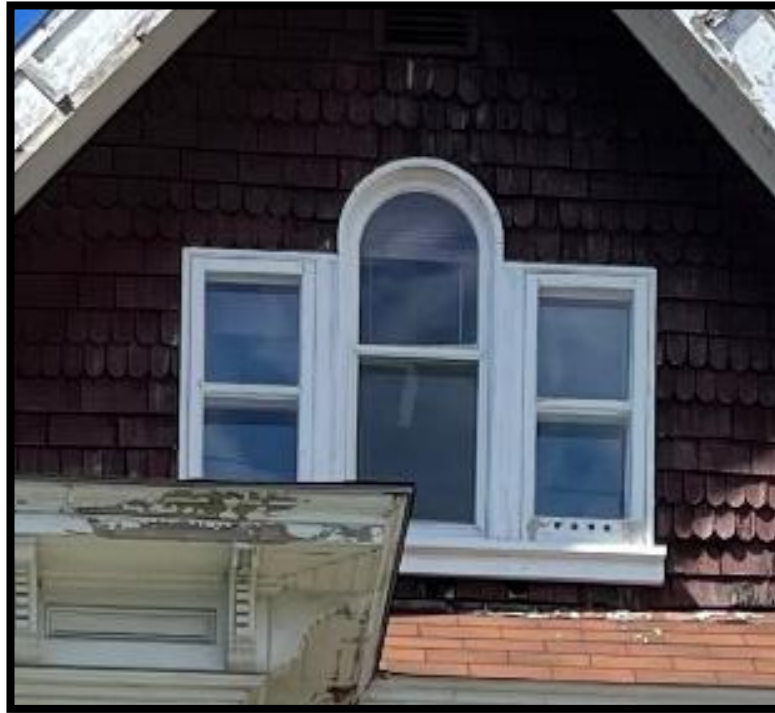
Figure 13: Palladian-inspired window in the attic of 366 Winona Avenue. The window is a simple configuration of two shorter and rectangular windows on either side of a taller round-headed window. It has no capping entablature connecting the set of openings. Credit: Matrix Heritage.
