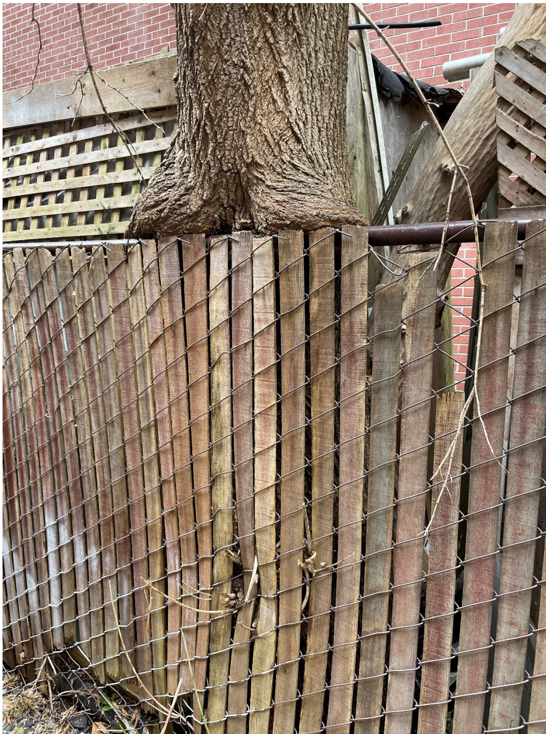
Figure 3: Tree 2, close-up of trunk growing into metal fence
