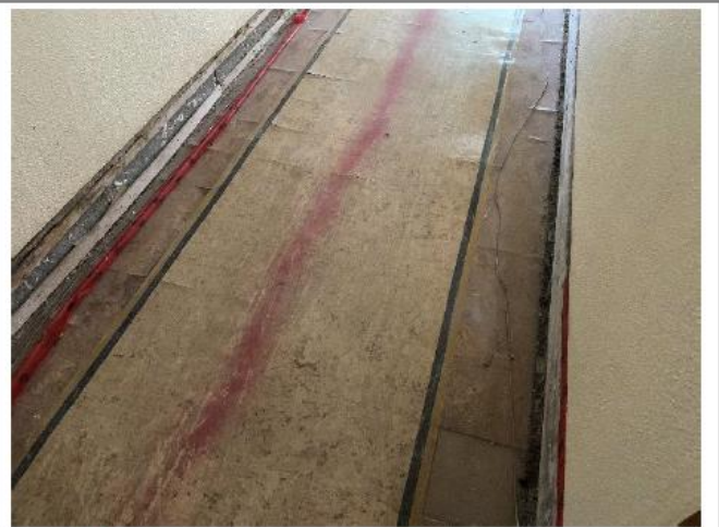
Figure 27: Extensive trim removals
