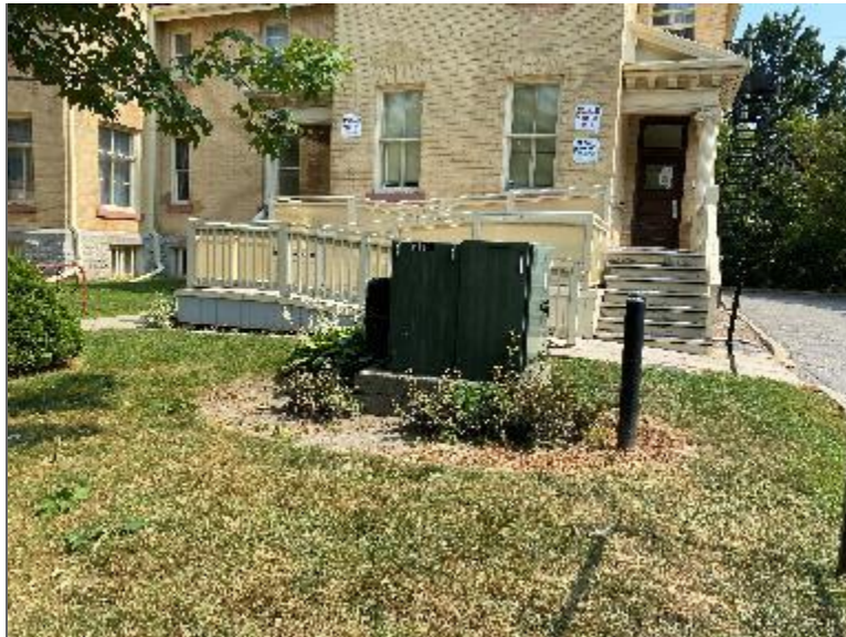
Photo 8 – Pad-mounted oil-cooled transformer located at the adjacent property northwest of the Phase One Property (PCA).
