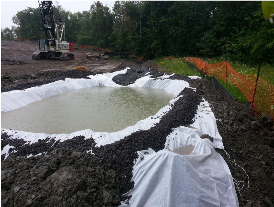
Photograph No. 1 – Photograph of the temporary retention pond 1 (Cell 1) located at the rear of Lots 5 and 6.
