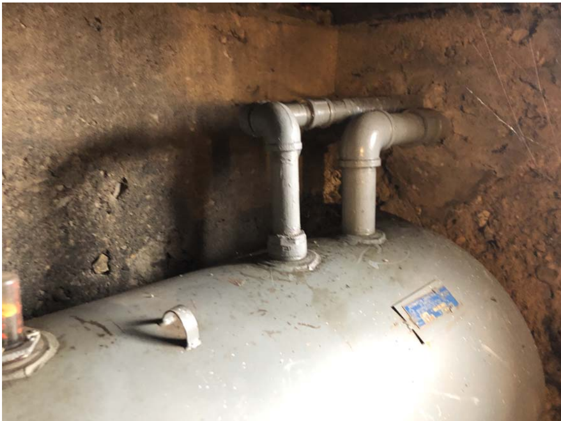
View of above ground storage tank within basement
