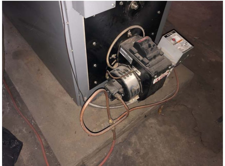
View of furnace within basement
