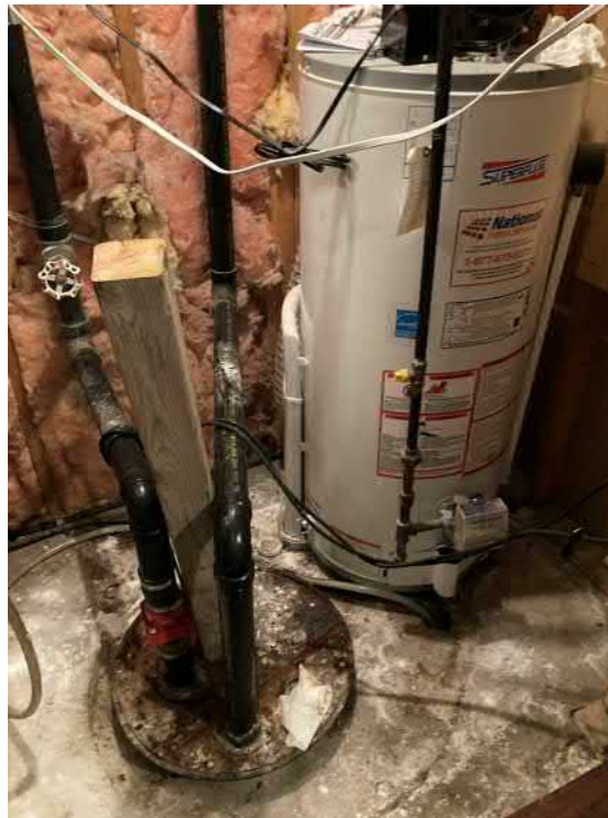
Photo 1: Sewage collection pit and water heater located in basement furnace room
