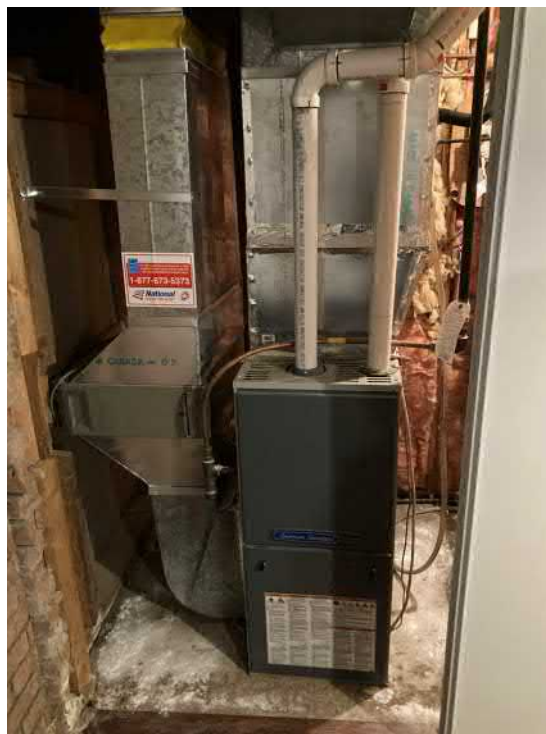
Photo 2: Gas-fired furnace located in basement furnace room
