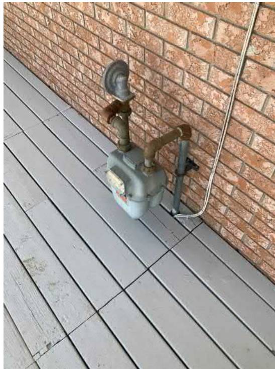
Photo 3: Gas connection on east side (front) of house
