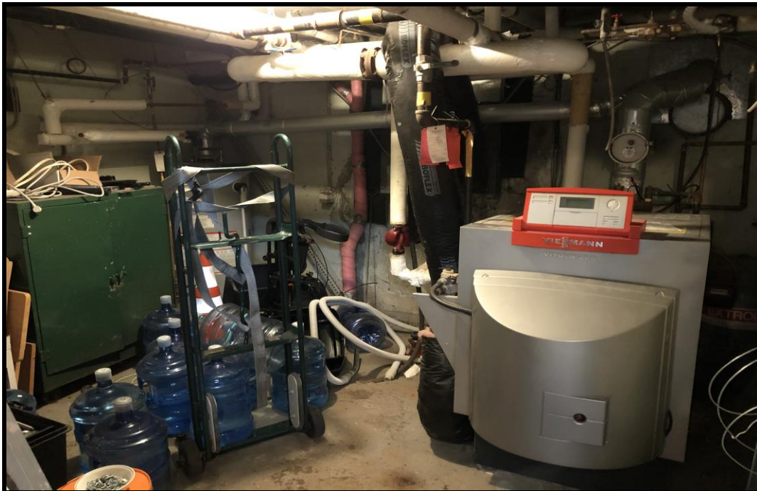
Photograph 6: View of the natural gas-fired boiler heating system, located in the basement of the curling arena at 2026 Scott Street.
