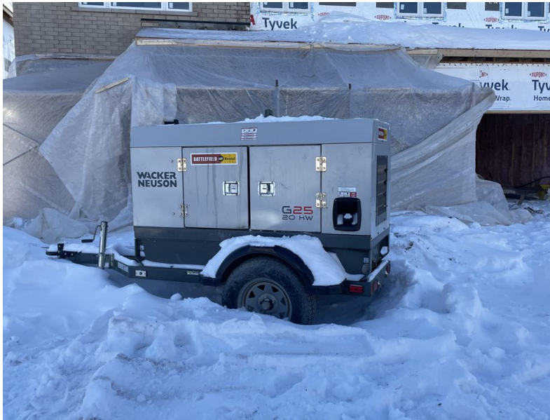
Photo 15 - Generator in the construction site south of the Site
