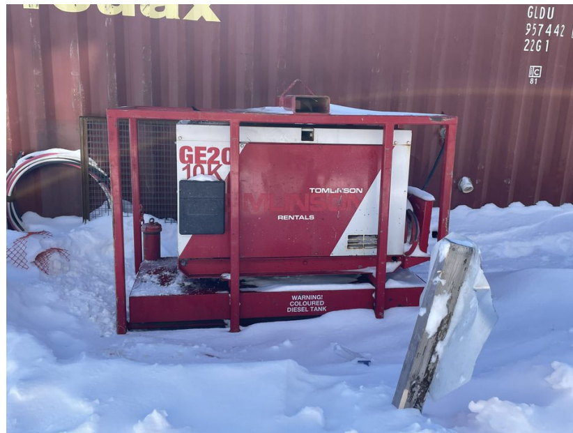
Photo 16 - Generator in the construction site south of the Site
