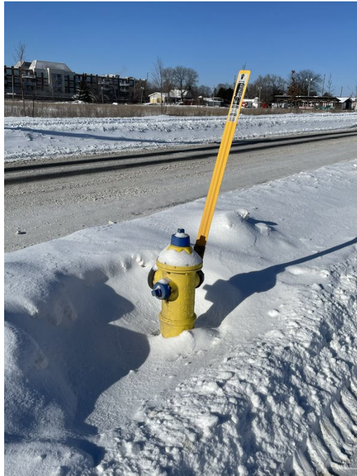
Photo 13 - Fire hydrant immediately to the west of the site along Lamarche Ave
