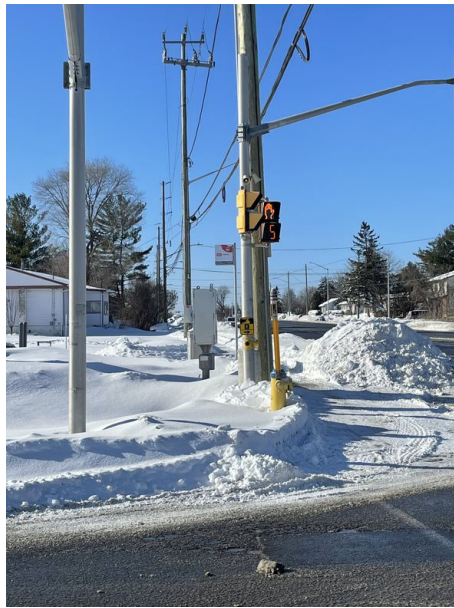
Photo 5 - Utility lines located on Innes, including a transformer
